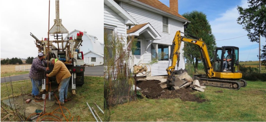
(Photos: Drilling the new well at the Kampen Road residence, by Mark Martin. Louis Meister tearing out the old masonry work at the Prairie Lane residence, by Maddie Dumas.)
